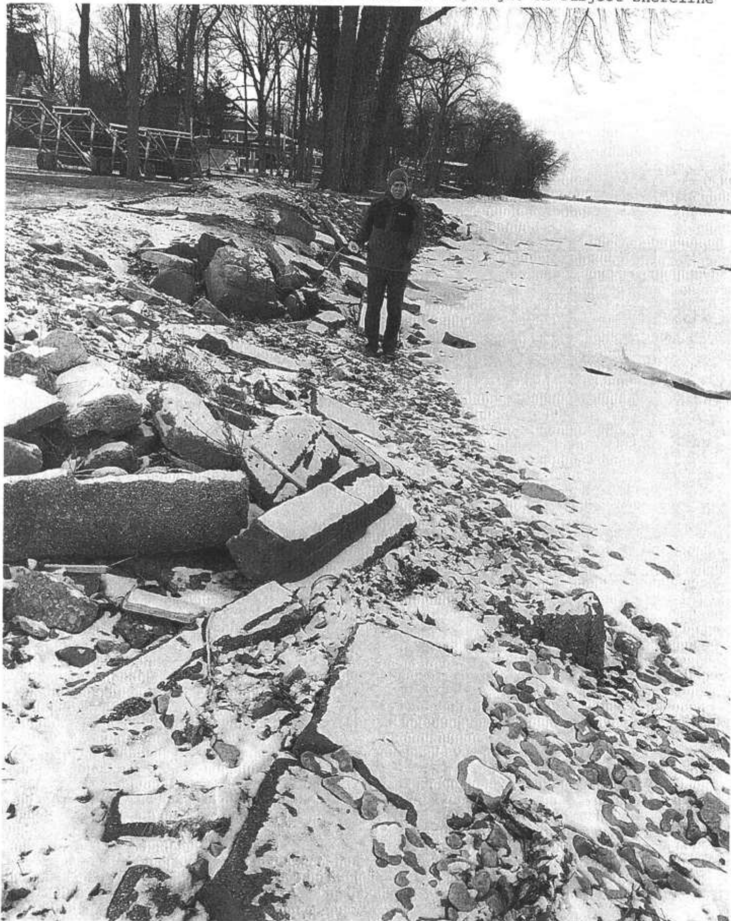
John Donnelly with cracked concrete "rock" on his right on subject shoreline
