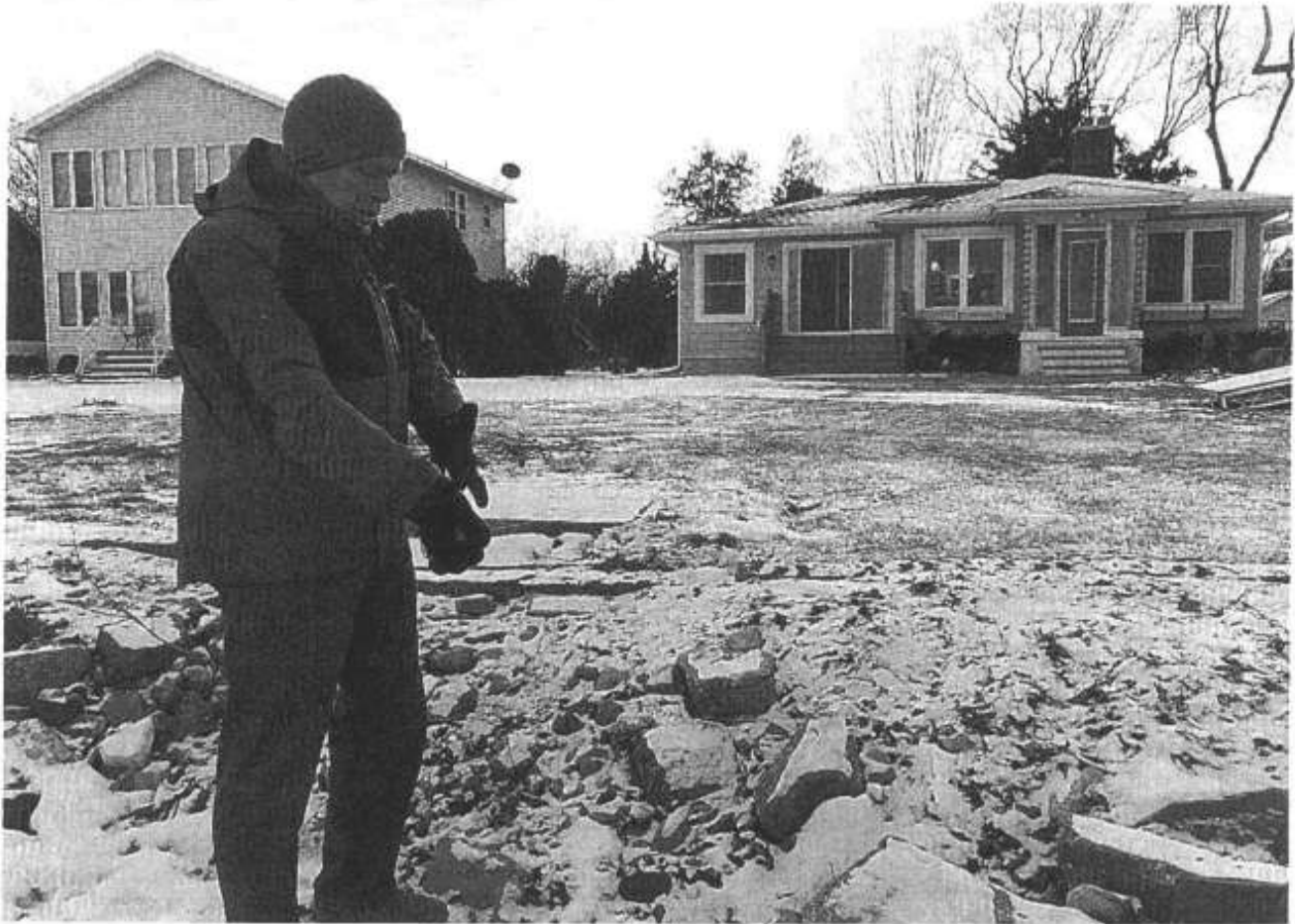
John Donnelly standing in front of subject property with cracked concrete "rock" to his right approximately 74' from the subject residence with patio at ground level in front of steps on residence.
