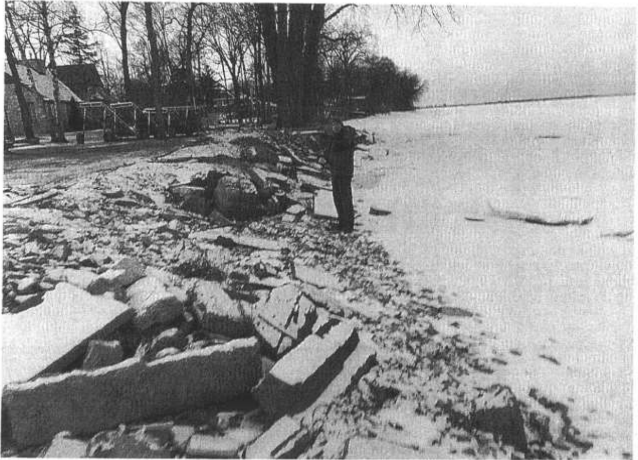
John Donnelly with cracked concrete "rock" approximately 4' to his right on subject shore line showing that set back from the principal structure on subject property is greater than 75' from the ordinary high water mark.
