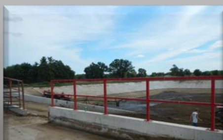
sand lane and outlet into manure storage
