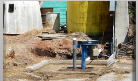
first flush leachate pumping system
