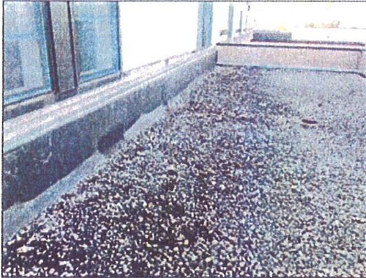
Membrane shrinkage on RA 7
