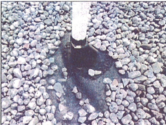
Membrane shrinkage on RA 18
