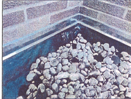
Flashings tenting on RA 7
