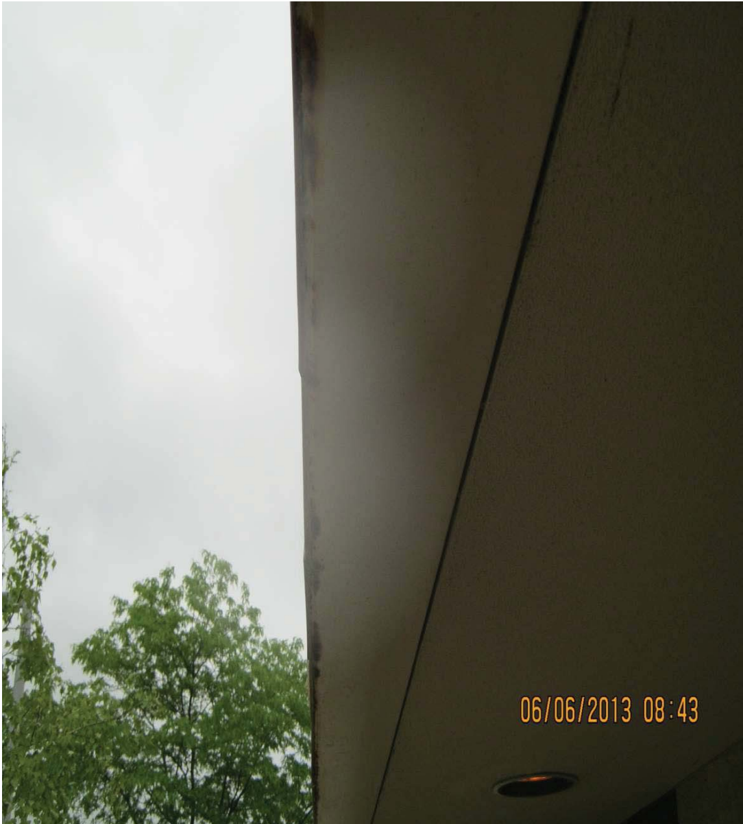
Highway Shop water damaged façade
