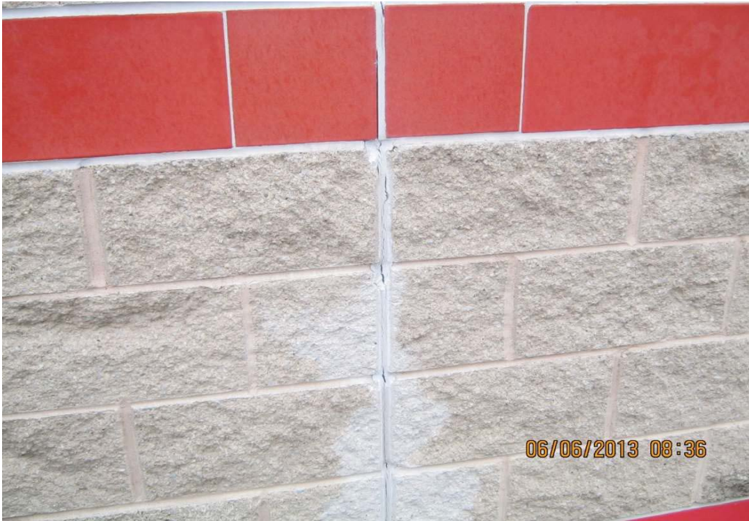
Highway Shop failed mortar joints
