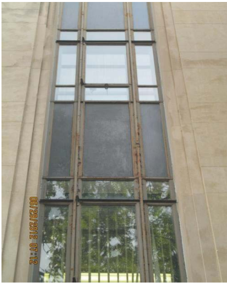
Rusting frames, discolored glass
