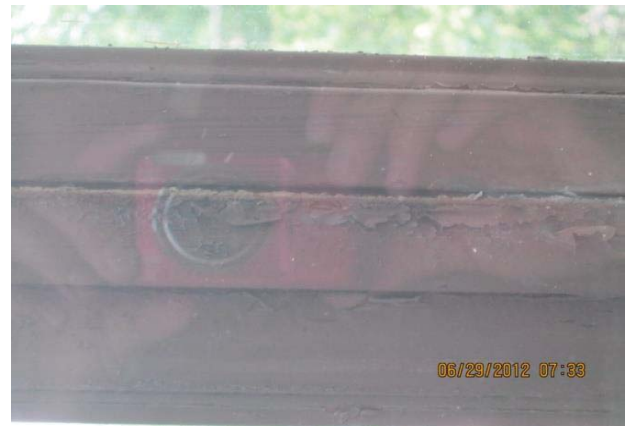
Interior framing corrosion
