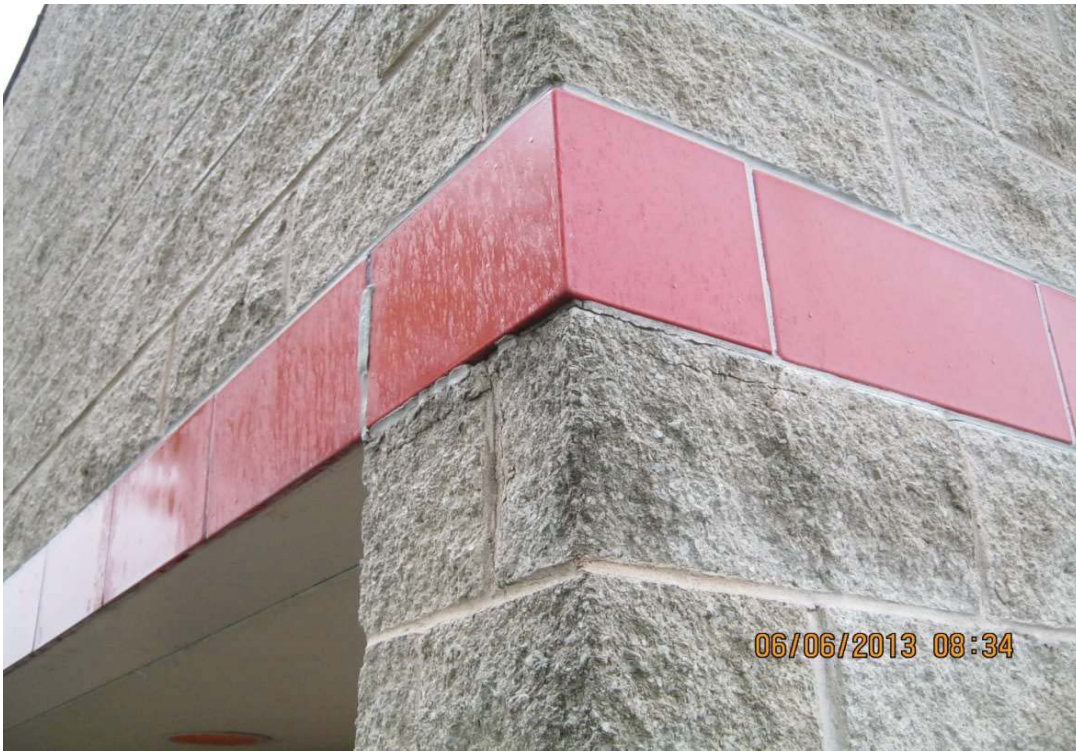
Highway Shop failed mortar joints
