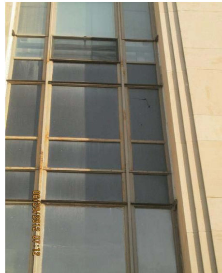
Glass is breaking due to corrosion in frame compressing the glass
