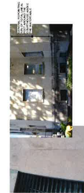
7. EXAMPLES OF GENERAL REPOINTING 10% OF TOTAL LINEAL FEET AT WINDOW SILL, COURTHOUSE AND THE WATERFALL
