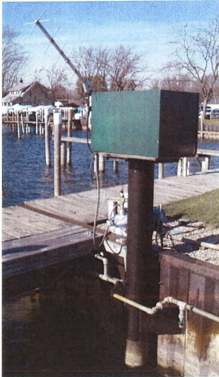
Photo of a Typical Water Level Gauge
