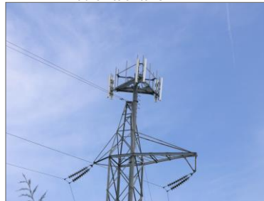
Exhibit 3-1 An antenna array mounted on top of a transmission tower
